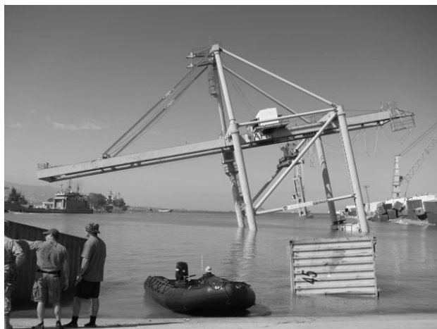
Figure 1. A failed container crane in Port au Prince, Haiti after the January 2010 earthquake [after Eberhard et. al., 2010]
